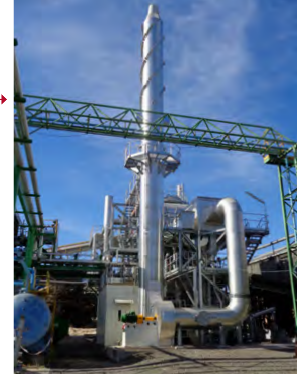
On-site energy centre →
